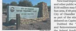
LEFT: Water treatment improvements are on the list of projects the City of Chandler is asking for federal funding for. In the background, water pipes and steel rebar to improve water supply.
